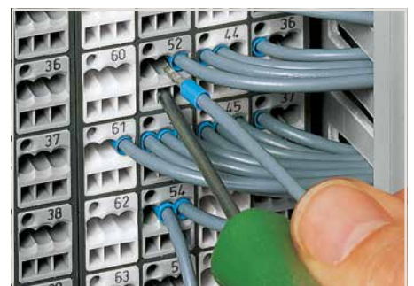
Terminating ferruled conductors via operating tool.
