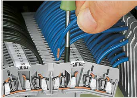
Terminal blocks for matrix patching: Inserting/removing a conductor in the terminal block's center.
