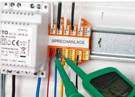
Testing via test ports opposite to conductor entry.
