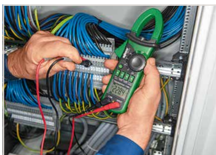
Current measurement in a switchgear cabinet
